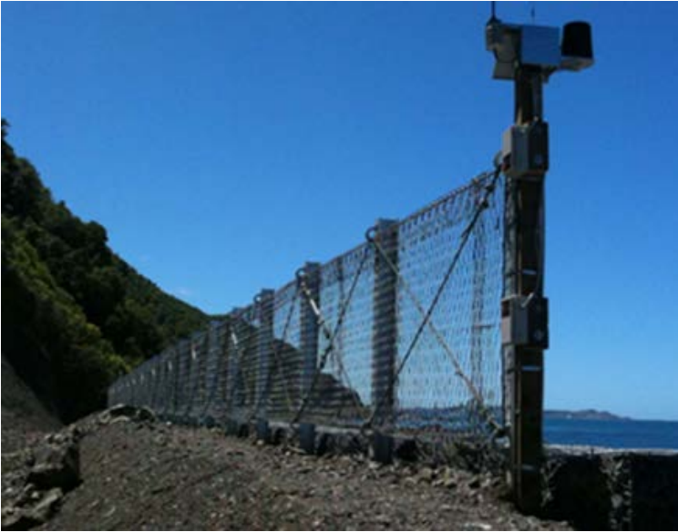
Figure 7.2 Tripwire system mounted to rockfall arrest fence (Source: NCTIR)
