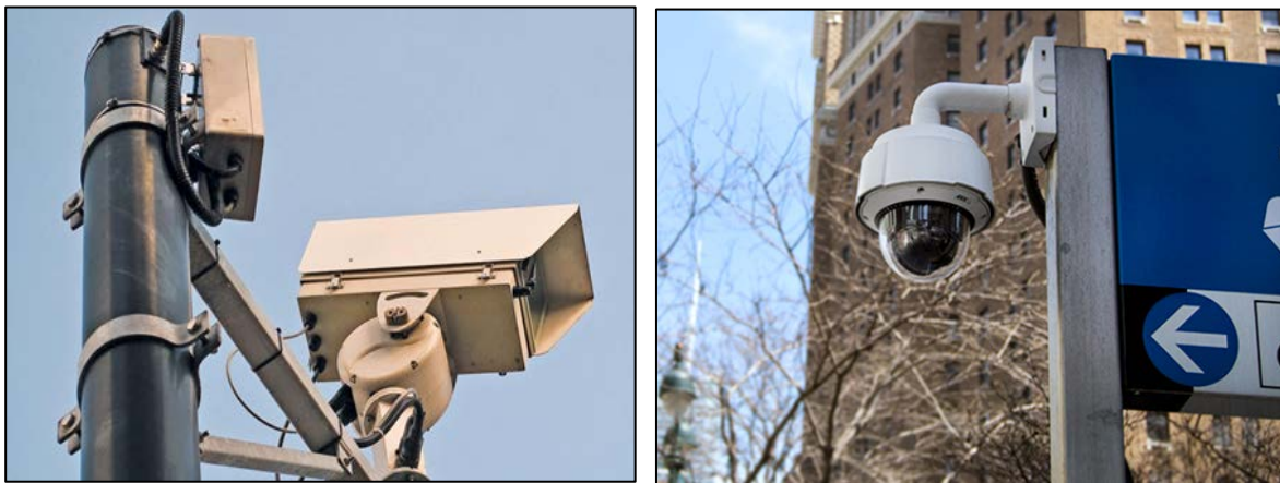
Figure 3.11 Examples of CCTV cameras (source: Auto Express and Axis Communications)
