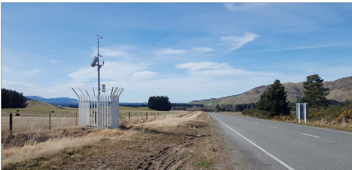
Figure 3.16 Roadside weather station near Porters Pass, State Highway 73 (source: authors)
