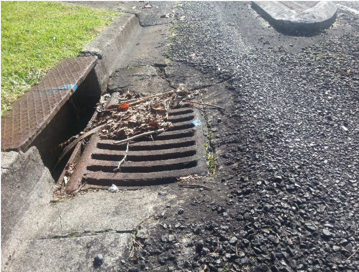
Figure 4.13 Note drop off into catch pit, greater than 5mm
