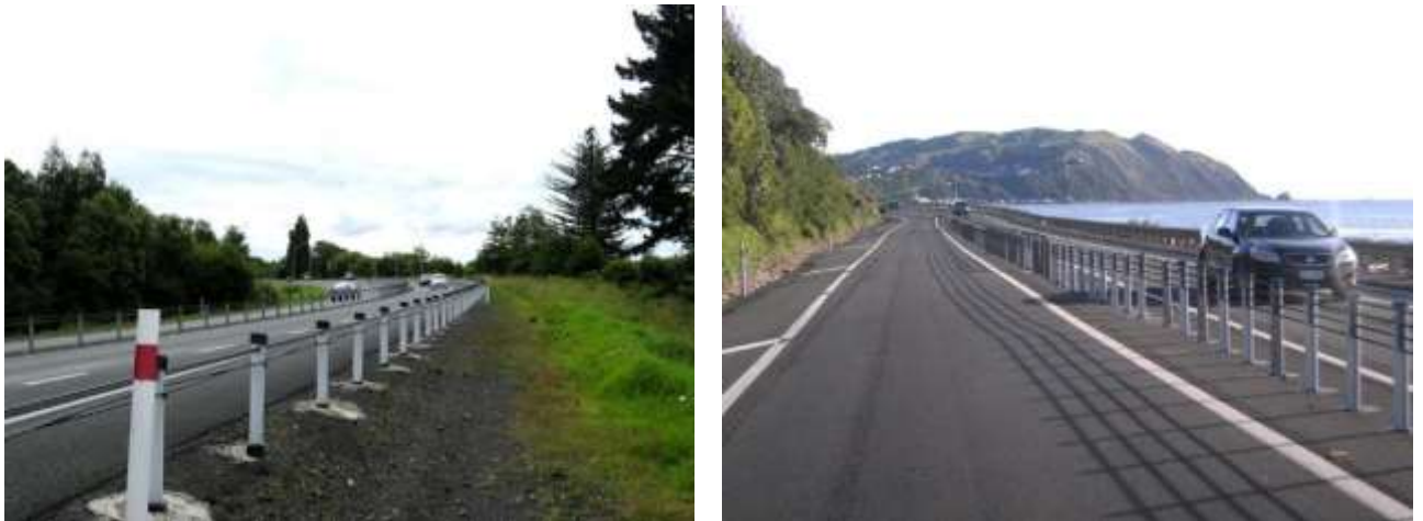
Figure 2.1 Wire rope barriers
