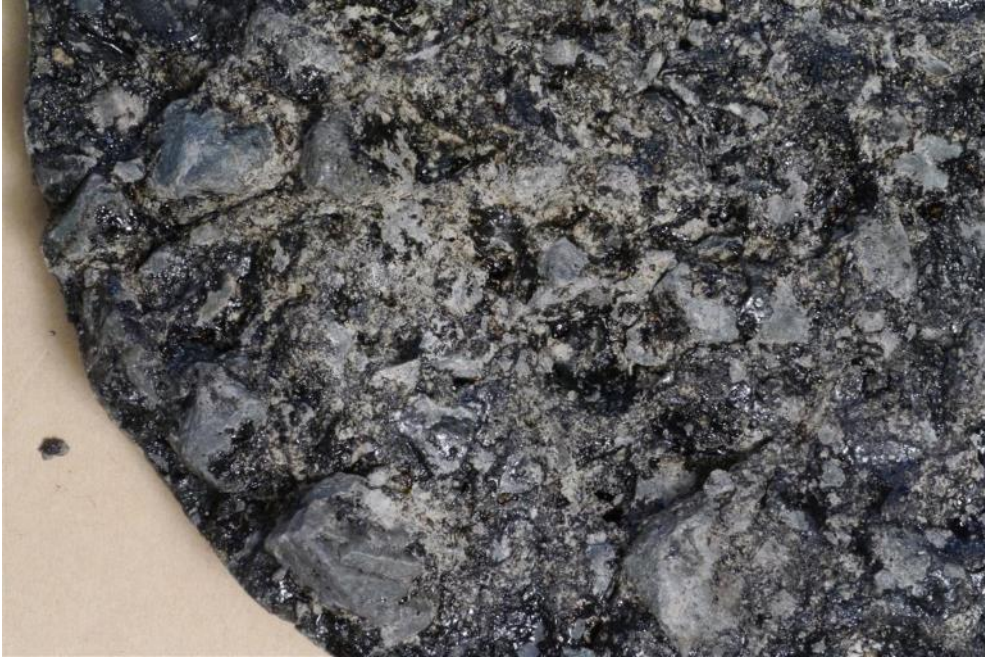
Figure 2.61 Site 6, base of core 10 (flushed patch) showing stripping
