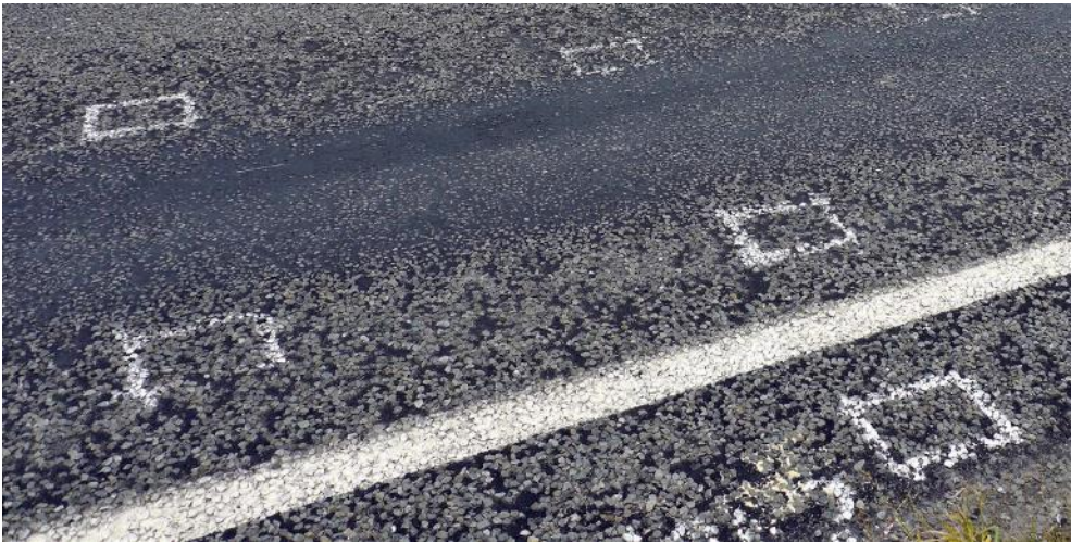
Figure 2.21 Blisters forming on the road shoulder as well as in the wheel path (SH75 Banks Peninsula)
