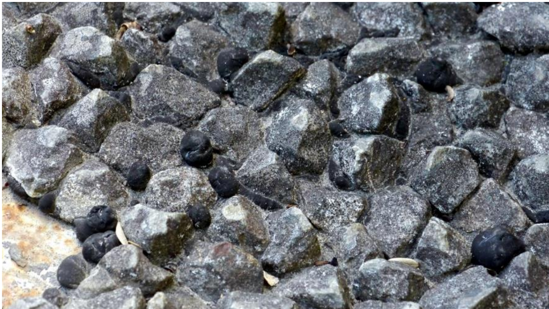
Figure 2.23 Bitumen blisters formed on an artificial seal constructed on a steel plate. The base plate is visible on the bottom left where earlier a sample had been removed
