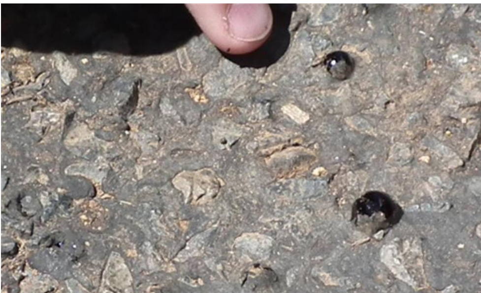
Figure 2.17 Bitumen blisters forming in hot weather (Melbourne, Australia)
