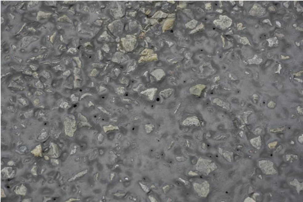
Figure 2.20 Water vapour vent holes in a flushed wheel track (SH2 Featherston)
