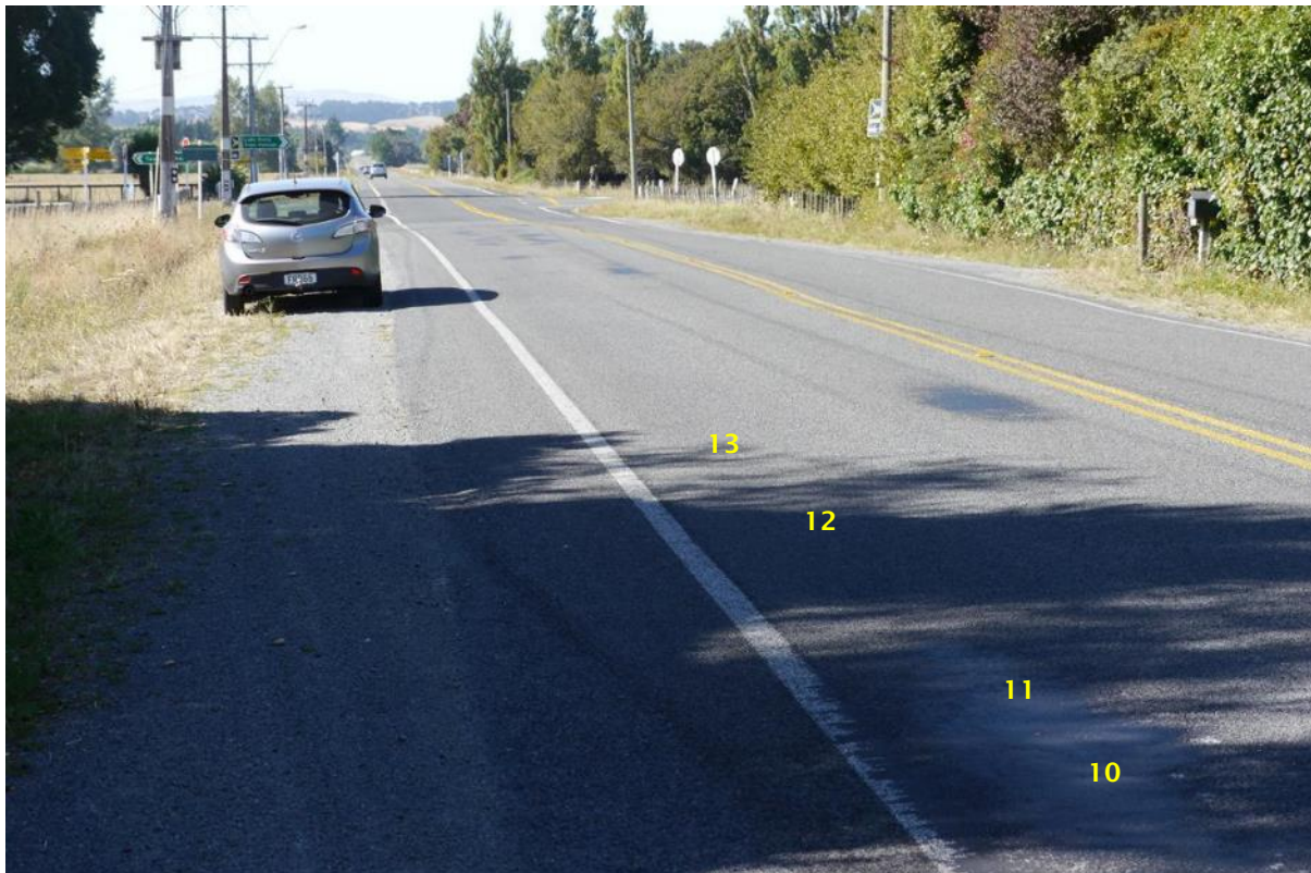
Figure 2.59 Site 6, flushed patch (in shade at bottom right)
