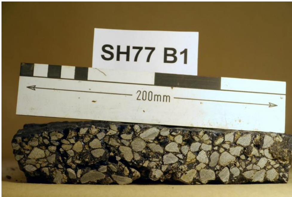
Figure 2.50 Site 4, specimen from flushed patch
