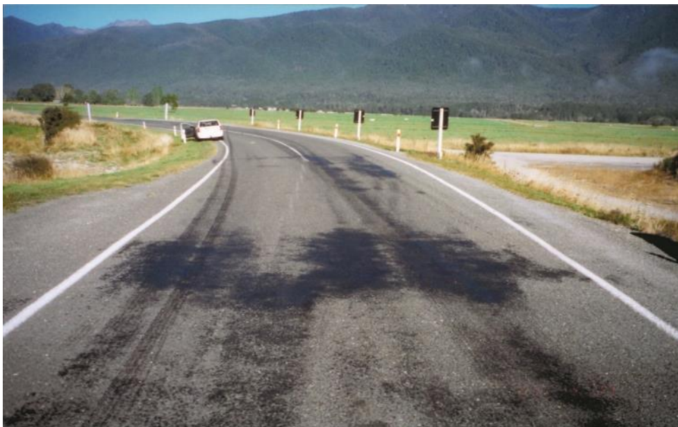
Figure 1.1 Seal with flushed patches and showing bitumen tracking in left wheel path
