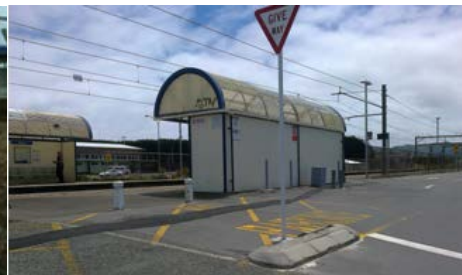
Mana station at the time of the survey had shelters with leaking roofs. The roofs have since been repaired and the subway repainted. (SB)
