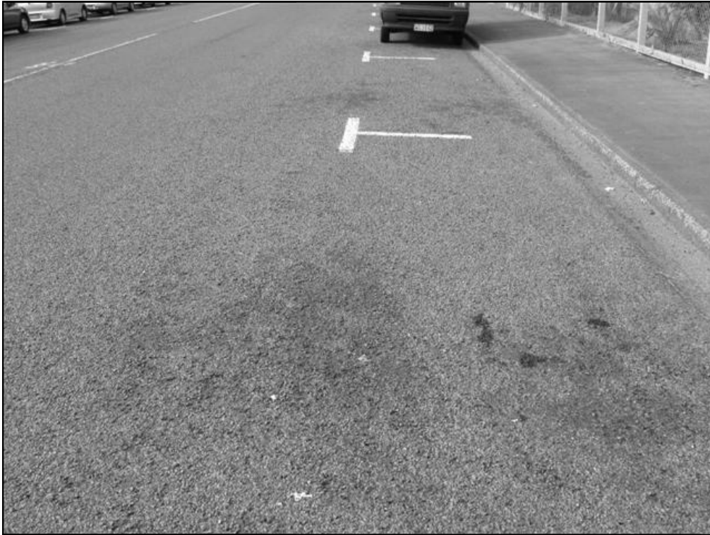
Figure 6.9 August 2009: chip loss in parking lane
