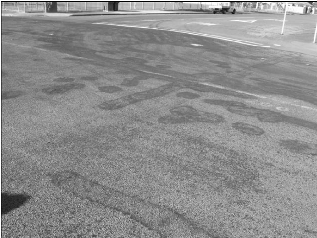
Figure 6.12 April 2011: repairs at the Lever Street-Domett Street intersection, with flushing also apparent in the multigrade bitumen seal (foreground)
