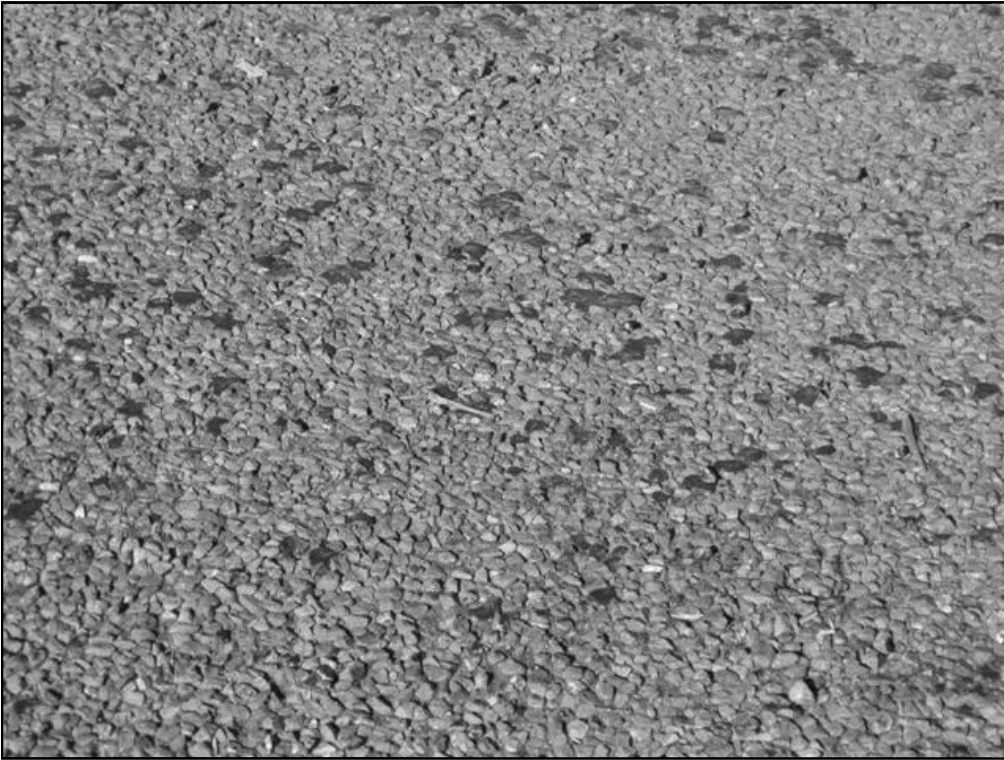
Figure 6.13 April 2011: spot flushing (venting) in the multigrade bitumen seal
