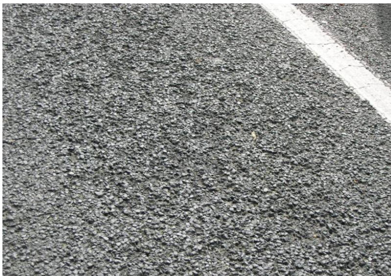
Figure 4.5 Ravelling due to ageing of the bituminous binder
