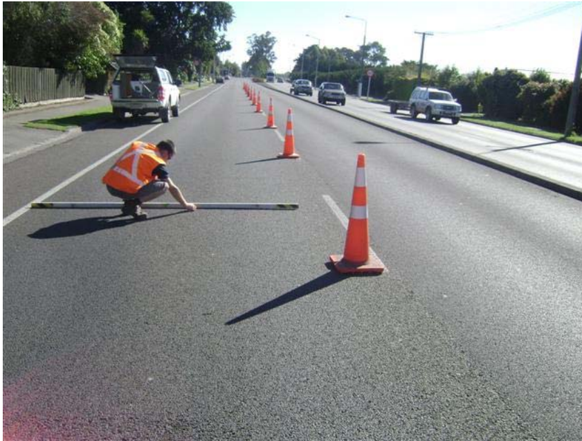
Figure 6.6 Start of 30% air void EMOGPA section, looking towards 20% air void OGPA section
