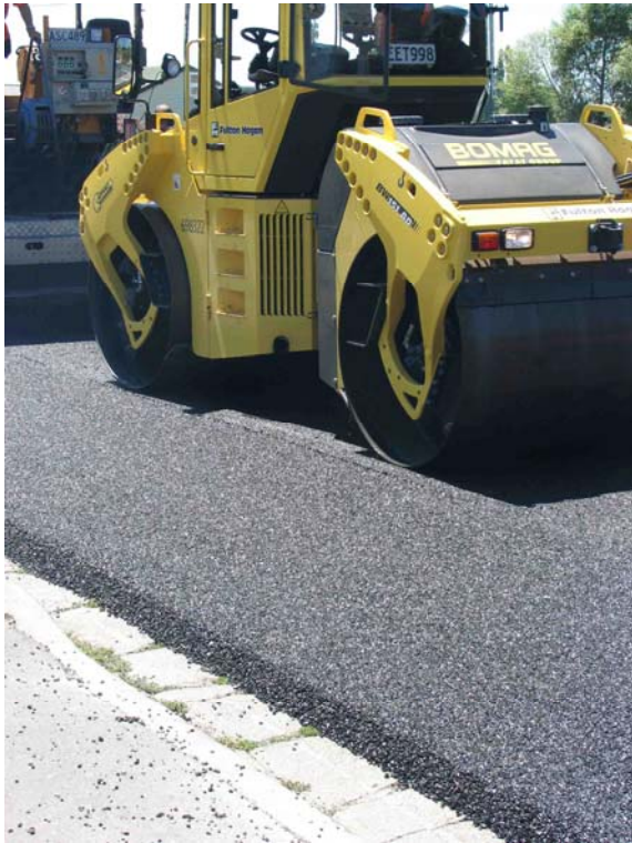
Figure 6.3 Compaction of the 20% EMOGPA section (plucked chip is visible outside the wheel tracks)
