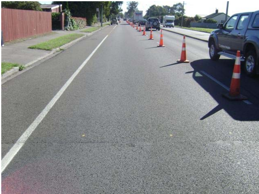
Figure 6.7 Start of 20% air void EMOGPA section, looking towards 30% air void EMOGPA section
