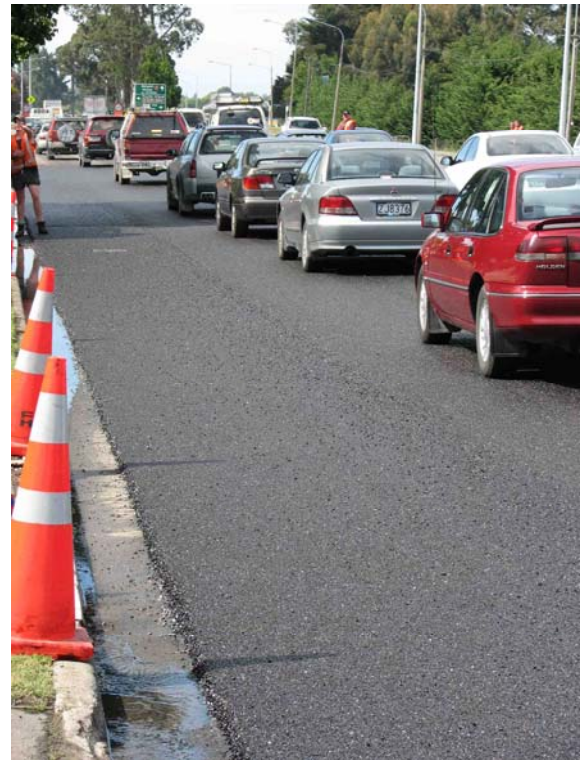
Figure 6.4 Traffic damage to the 30% epoxy OGPA
