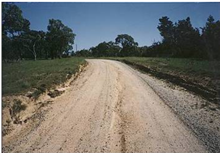
Figure 3.8 Longitudinal scour due to steep vertical grades.
