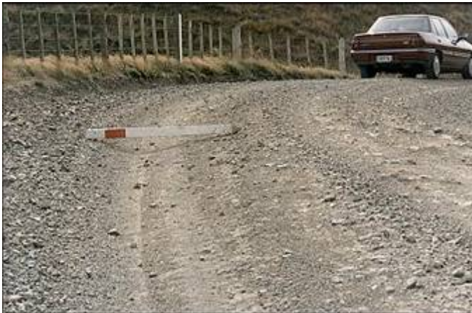
Figure 3.7 Tight curves with high road surface wear.
