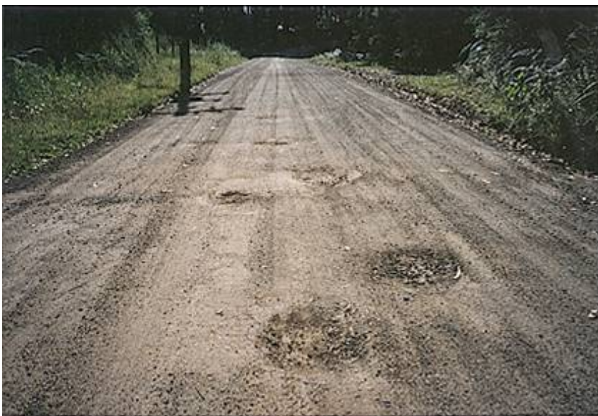
Figure 3.6 Creation of potholes due to flat crossfalls.
