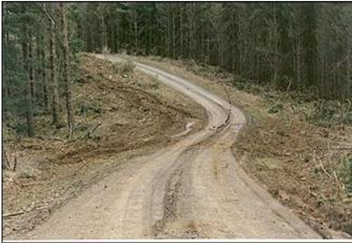
Figure 3.9 Soft spot developed on road surface due to poor horizontal/vertical coordination.
