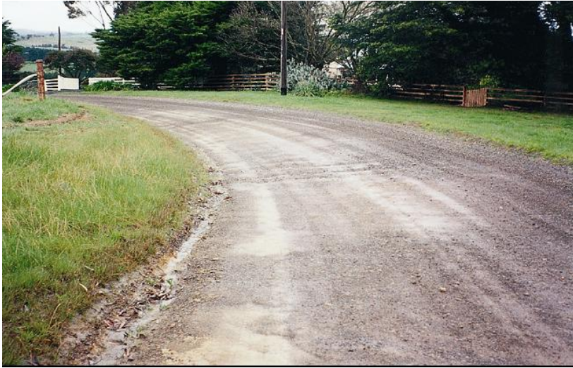
Figure 3.11 Transverse scouring on road.
