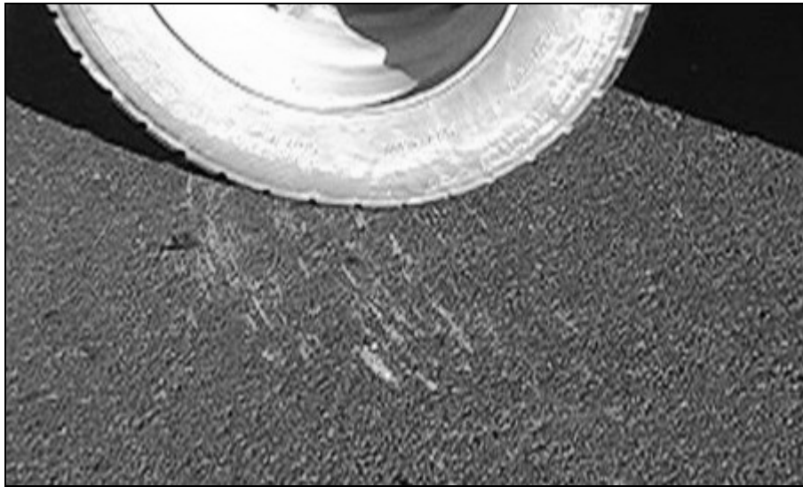
Figure 3.6 Pavement scuffing damage from the seven tonne experiment.
