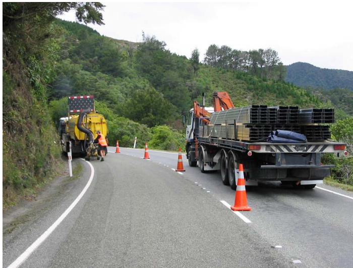
Figure 4.7 Watercutting at Whangamoia Saddle site.
