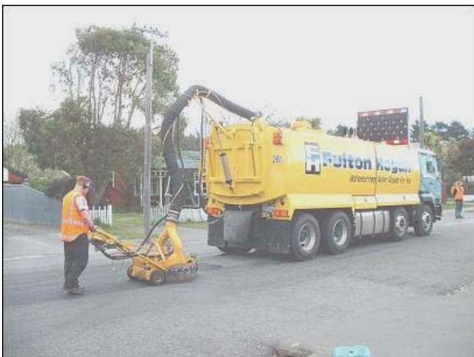
Figure 2.2 Water supply and vacuum recovery system.
