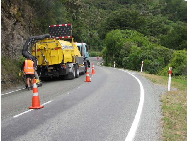
Figure 6.2 Flushed, rutted wheelpath on Whangamoia Hill site.
