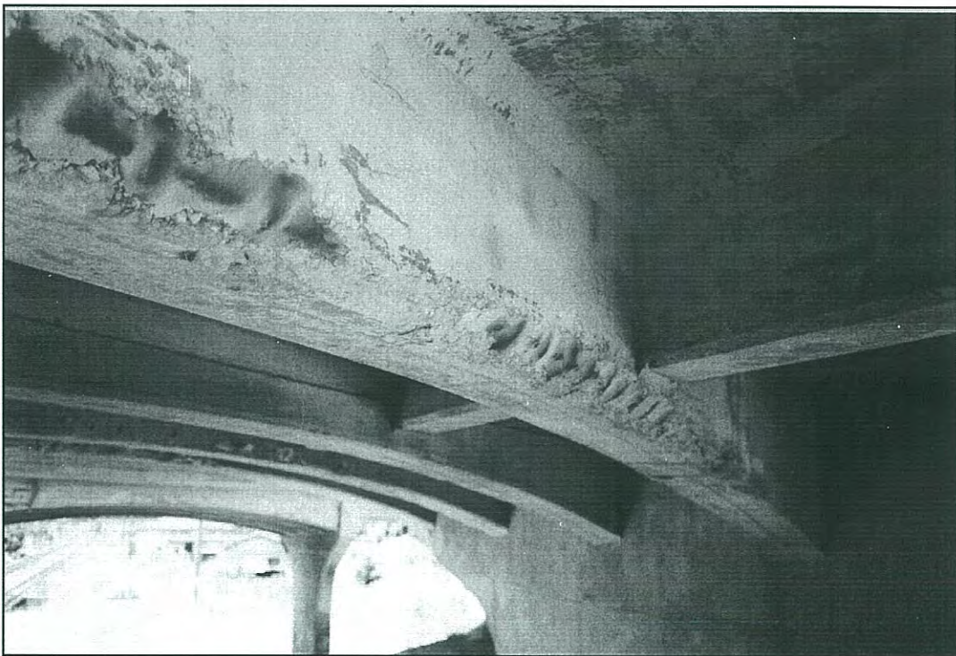
Figure 4.1 Epoxy patch repairs that have failed to prevent ongoing corrosion.
