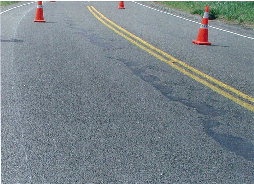
Figure 5.3 Scabbing on Harcourt Werry Drive at 300 m in the RWP.
