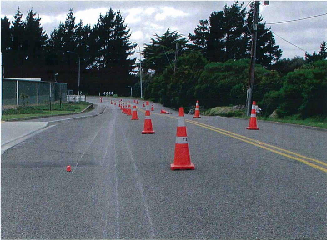
Figure 5.2 Site start, approach to first corner on Harcourt Werry Drive. Note seal patch from kerb.
