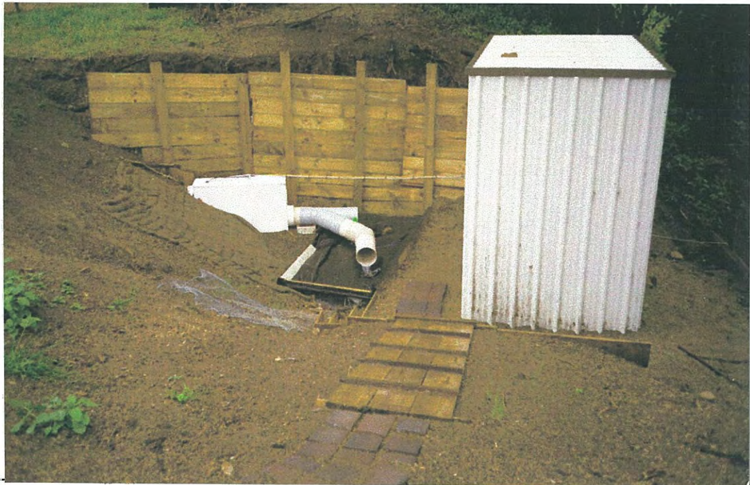
Figure 3.5 The experimental site with the installed equipment.
