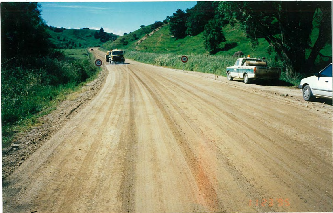
Photo 3 (upper): Section 1 23/11/95 Final shaping of surface - several light passes by the grader were required to bring sufficient fines to the surface. Photo shows grader followed by vibrating roller (Sakai SU700, 7.2 tonne).
