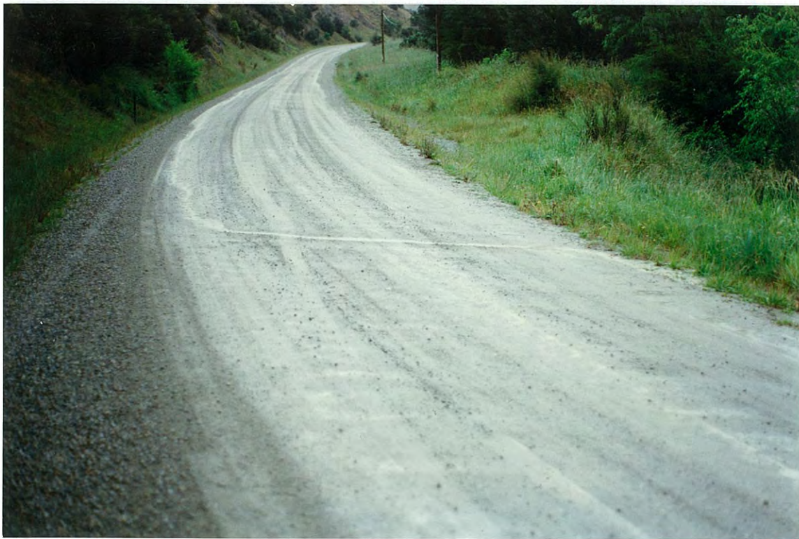
Photo 13 (upper): Section 1 Shallow shear failures causing severe loss of shape within section 1.
