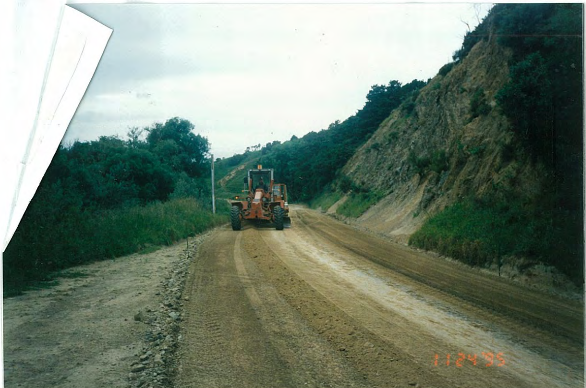
Photo 1 (upper): Section 1 22/11/95 Close up of rotary hoe (Sakai PM170 fitted with carbide tines) mixing Endurazyme into pavement material. Note very fine tilth behind hoe.
