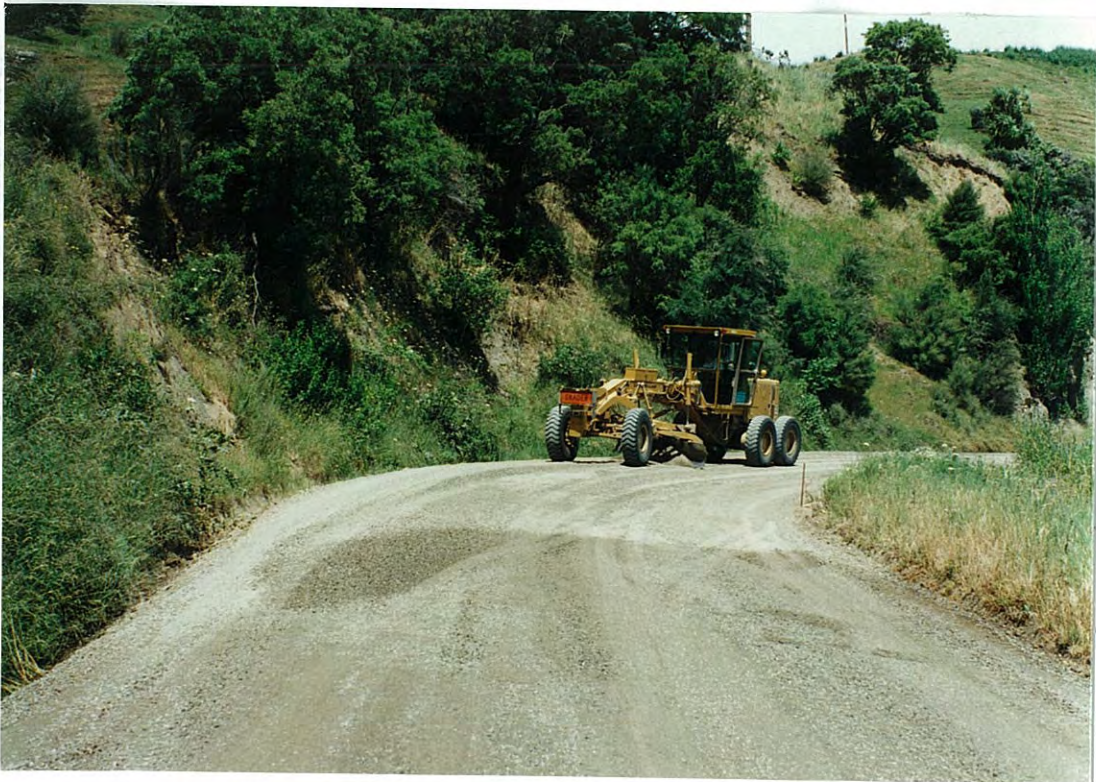
Photo 5 (upper): Section 4 Placement of granular wearing course using truck and trailer units.
