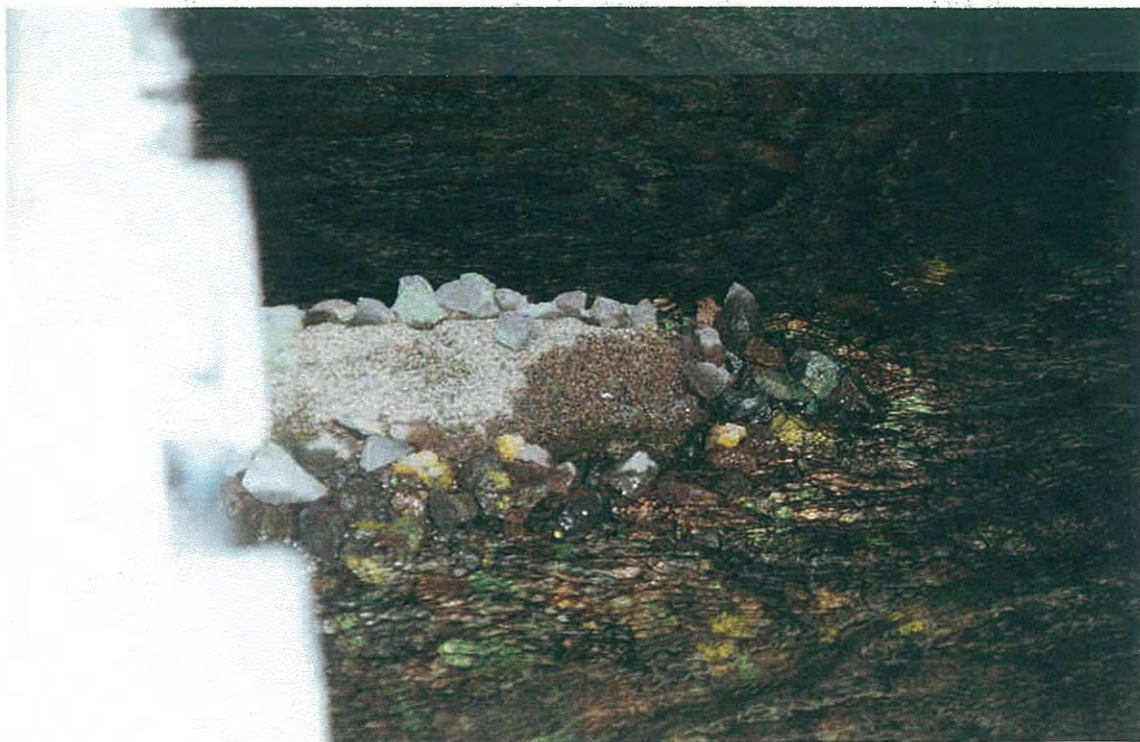
(a) Catastrophic rapid failure (no filter fabric).
