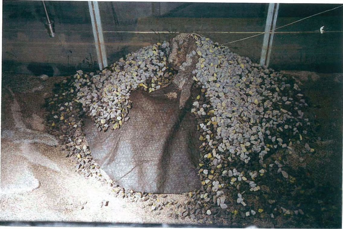
(b) Failure due to exposure of the filter fabric at the abutment toe, allowing slumping of the sand embankment.
