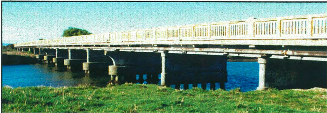
Figure 3.1 Waitangi Washout Bridge, in Hawke's Bay, North Island, New Zealand.
