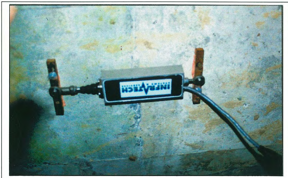
Figure 4.3 Demountable strain gauge over a crack in the slab.
