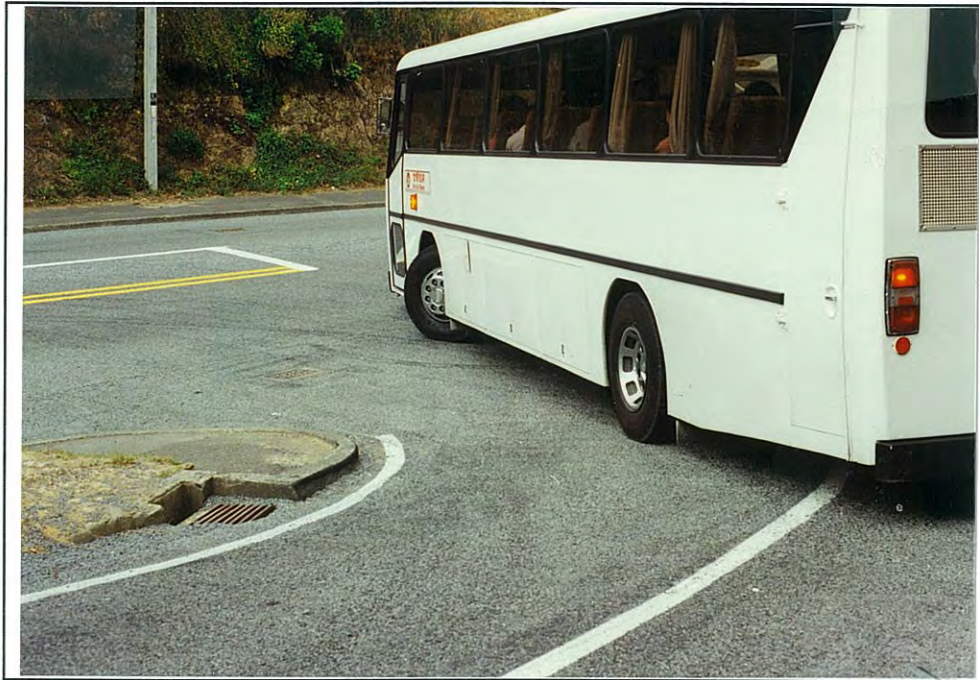
Figure 6.4 This bend on Crawford Road, Wellington, showed no traffic-related distress after one month.
