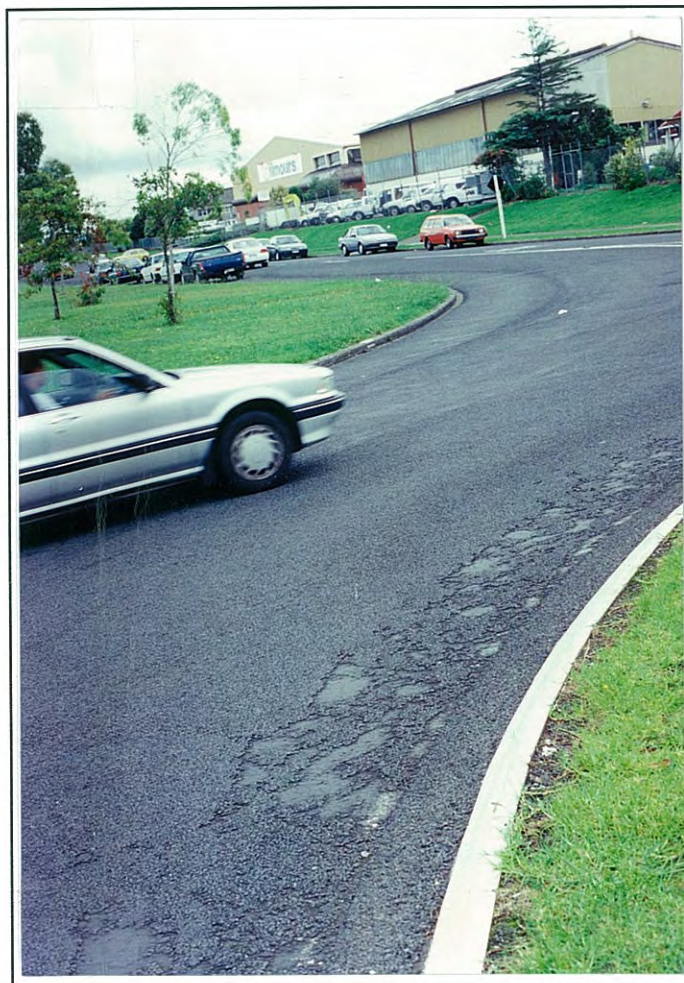
Figure 6.1 Distress after one year at Lambie/Cavendish roundabout, Auckland.
