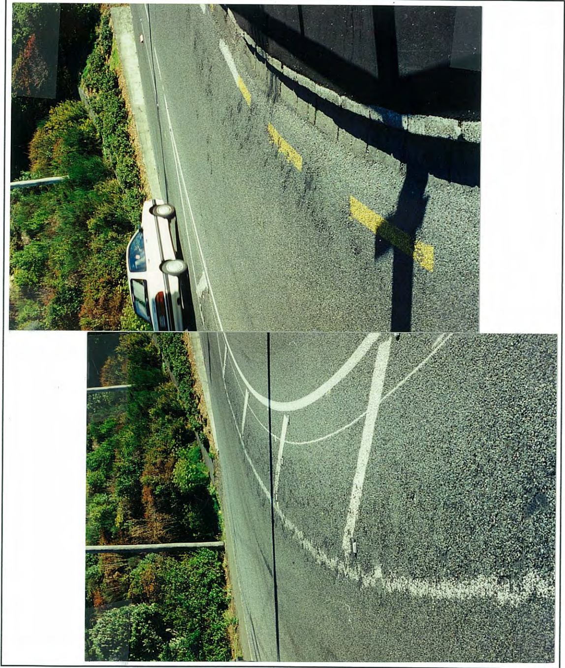
Figure 6.6 Detail of distress on inside bend of Crawford Road, Wellington, after one month. a. Uphill lane b. Downhill lane
