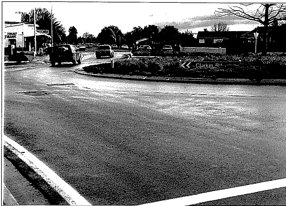
Figure 3.1 Centre of roundabout showing 20% WODB section (foreground) and control section adjacent to roundabout hub, at beginning of trial.
