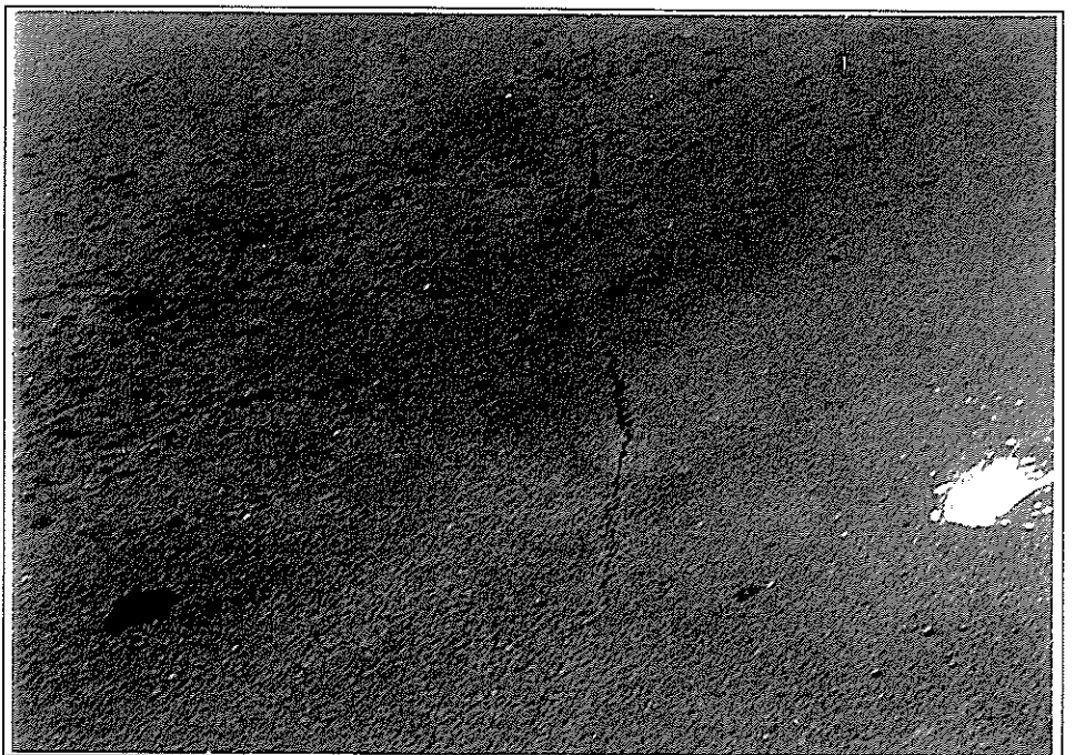
Figure 4.3 Transverse and longitudinal joint between the 9% WODB section (on left) and control section (on right) after 57 months.
