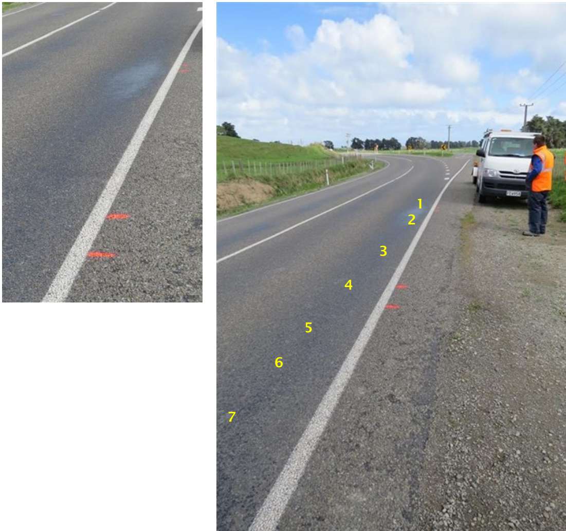
Figure 3.11 Cracked and flushed seal site (SH57 Shannon) showing core sample positions
