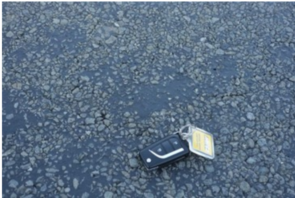
Figure 2.3 Cracking is very often associated with flushing
