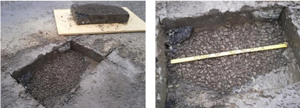
Figure 2.11 An example of a slab cut and removed from the SH1 site (left); in this case the slab partially delaminated leaving behind part of the first coat seal and was not used.
