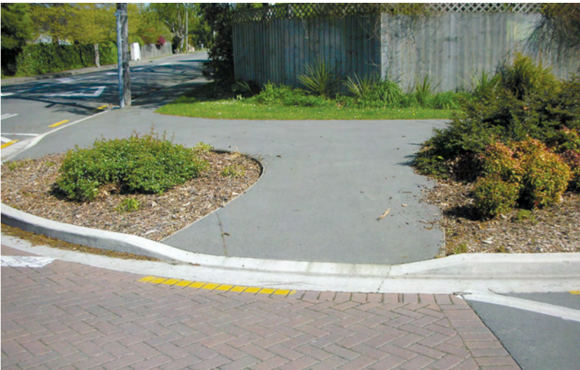
Photo 6.10 – Kerb ramp, Christchurch (Photo: Megan Fowler) (note: missing tactile paving)
