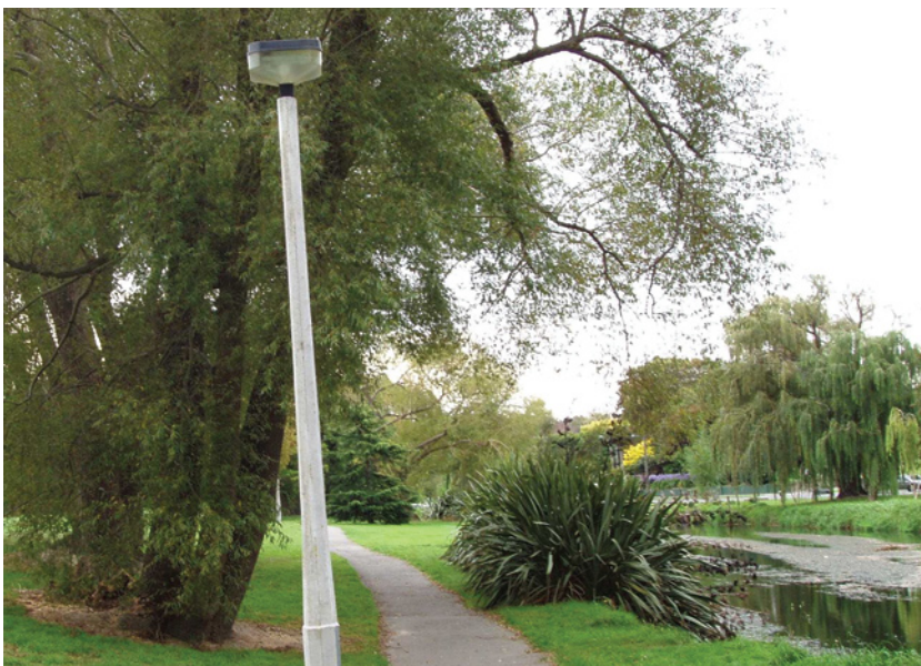
Photo 17.2 – Medium height lighting column, Christchurch
