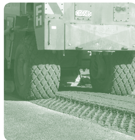
The in-situ recycler at work during the study stabilising the contaminated material.
