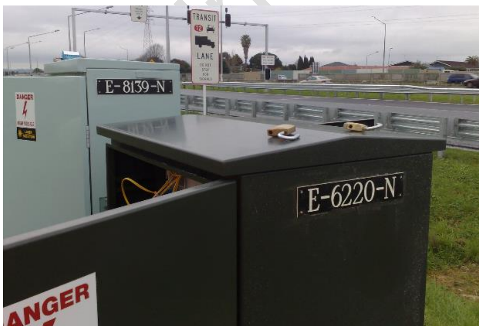
Figure 2: Communications cabinet E-6220-N and ramp signals cabinet E-8139-N with their identification labels facing the approaching traffic
