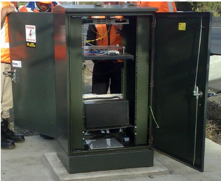
Figure 4: Rear of a cabinet
