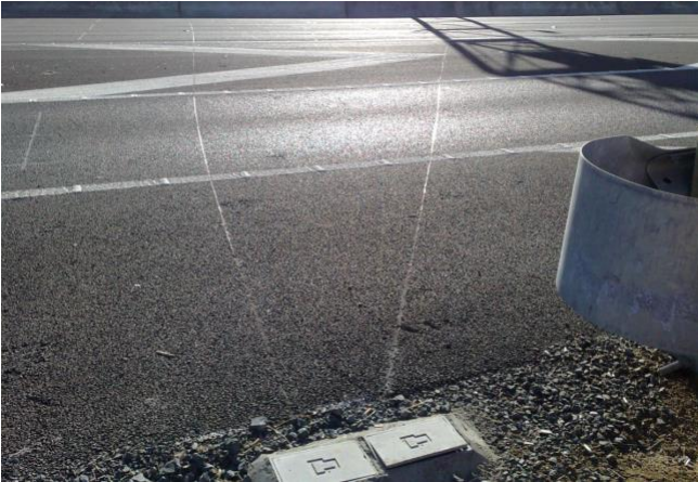
Figure 7. The loose lid of traditional traffic signal cable jointing boxes can form dangerous projectiles in high speed locations and must not be used
