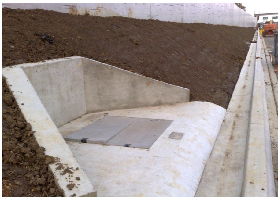
Figure 10. Example of a double jointing chamber and a hinged galvanised hinged steel 250mm x 170mm cable jointing box constructed into a steep slope.
