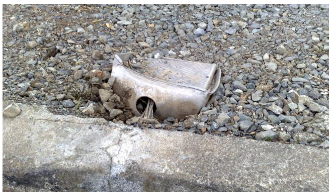
Figure 6. The importance of securely concreting a cable jointing box into the ground is demonstrated in this illustration
