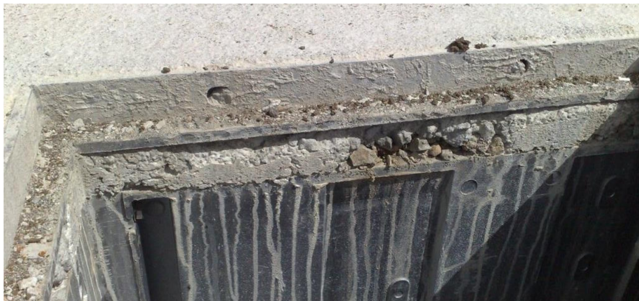
Figure 3. Over-concreted and poorly installed coverset frame with concrete on the seating lip and in the locating holes.
