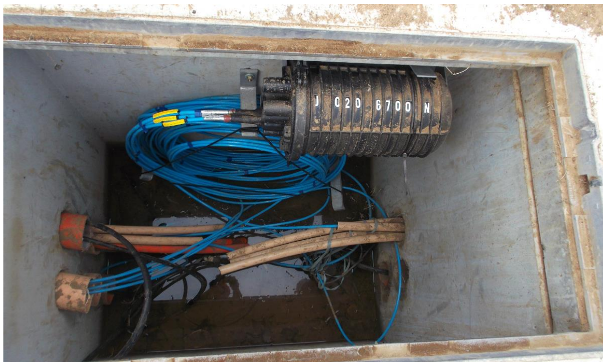
Figure 1. Example of a 1200mm x 900mm jointing chamber with a 1200mm x 600mm coverset. The joint is attached to a wall mounted bracket and there are cable management brackets attached to the same wall. The backbone duct has protruding sub-ducts and the chamber also contains local fibres and detector/power cables.
