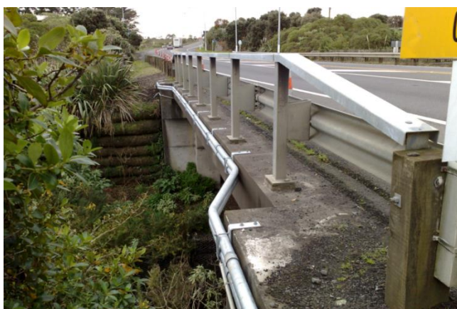
Figure 3. Typical galvanised steel ducting on the side of a bridge.
