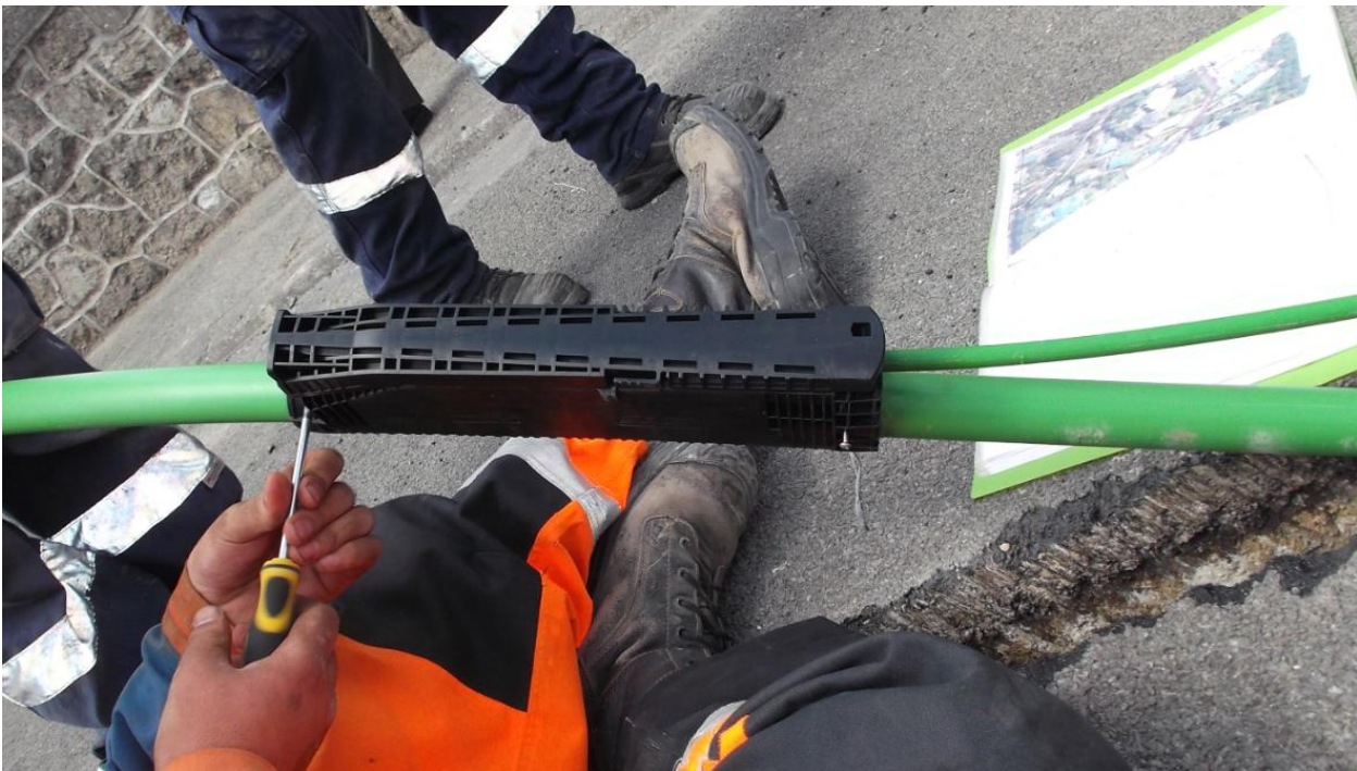
Figure 4. Example of a direct-buried ducting connector being installed. These connectors allow a spur to be broken out of the duct line. The spur itself is broken out from the backbone fibre at an upstream joint. The spur fibre is thus blown from joint to asset through this connector. This enclosure is direct-buried into the trench (visible on the right). These are green ultra-fast broadband ducts.
