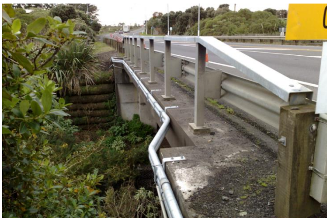
Figure 9. Typical galvanised steel ducting on the side of a bridge.
