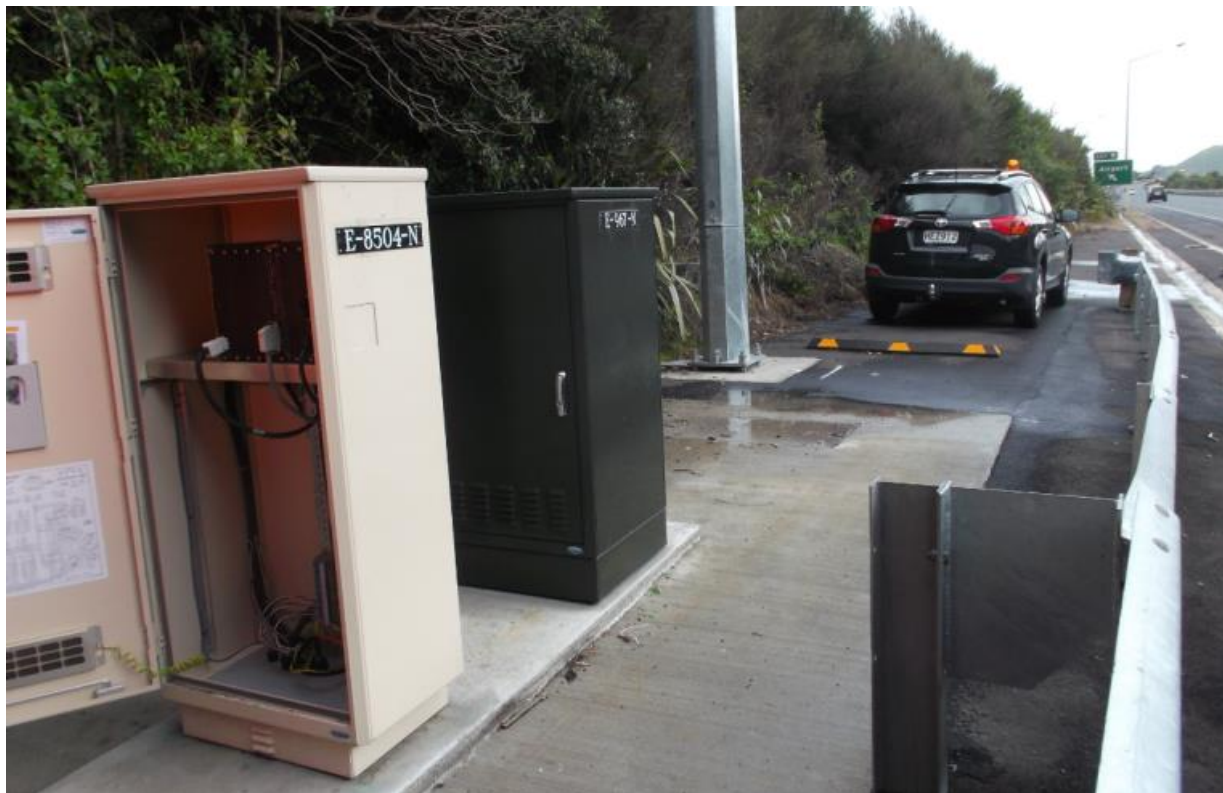
Figure 17. CCTV, communications cabinet and ramp signals cabinet on a constrained site. Note the bump stop for the reversing maintenance vehicle.
