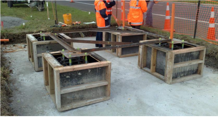
Figure 1. Cantilever gantry foundation under construction with steel templates for the holding-down bolts, the duct access and the spacing of the gantry legs.
