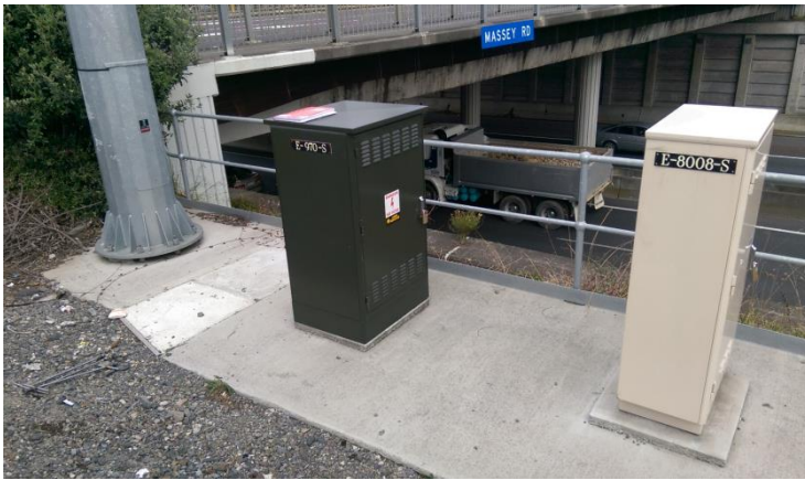
Figure 2. Lowering CCTV pole with communications cabinet and ramp signal cabinet atop a retaining wall with safety rails and a kickboard.
