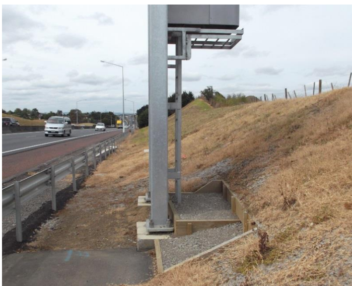
Figure 16. Safe ladder access to a VMS gantry.
