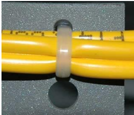
Figure 13. Cable tie is too tight.
