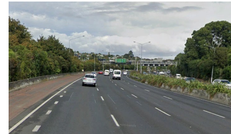
Concrete barrier within 5m of edgeline
