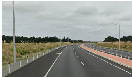
Wire rope barrier within 5m of edgeline
