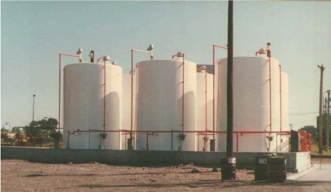
Figure 1 A typical small fuel tank farm
