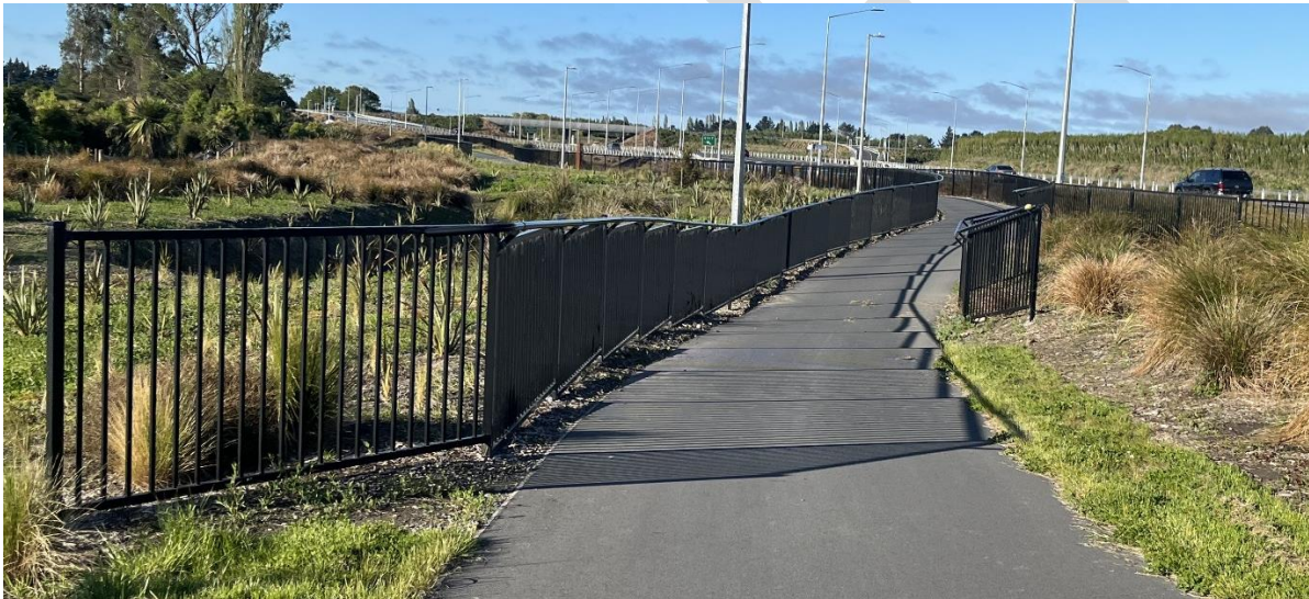
Railing flared out to mitigate snag risk, Christchurch Northern Motorway shared path (photo: James Wratt)
