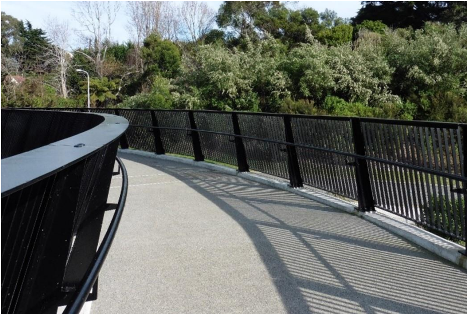
Inward leaning fence restricts visibility around corner and reduces useable width. Leinster Ave Footbridge, Kapiti (photo: James Wratt)
