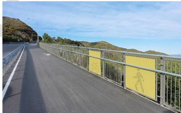
1400mm fence on a steep downhill gradient with curves. Wainuiomata Hill Shared Path (photo: James Wratt)
