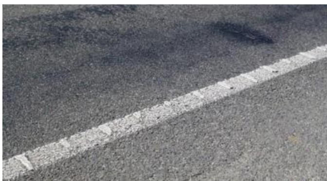
Figure 8-1: ATPM damaged by snow plough (Lester et al, 2017, page 34)
