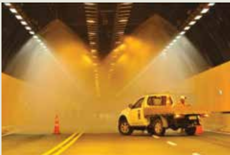
THE DELUGE SYSTEM - DESIGNED TO SUPPRESS A FIRE IN THE TUNNEL UNTIL THE FIRE SERVICE ARRIVES. WOULD DELIVER WELL OVER 3000 LITRES OF WATER A MINUTE IN THE EVENT OF A FIRE - THE EQUIVALENT OF 390mm PER HOUR.
