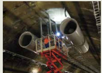
THE FANS - EIGHT NEW 90kw FANS, SIMILAR IN POWER TO A SMALL CAR, HAVE BEEN INSTALLED IN THE ROOF SPACE. ON A DAILY BASIS, THE FANS HELP MAINTAIN AIR QUALITY, AND IN THE EVENT OF A FIRE CAN BE USED TO CONTROL SMOKE BY BLOWING IT AWAY FROM THE SOURCE, ENABLING FIRE CREWS A BETTER VIEW OF THE FIRE, AND PROVIDING A CLEAR PATH FOR PEOPLE TO ESCAPE THE TUNNEL.
