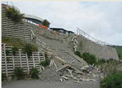
DAMAGE FROM THE FEBRUARY 2011 EARTHQUAKE - COLLAPSED CRIB WALL IN GALILEE LANE, SUMNER, CHRISTCHURCH.
