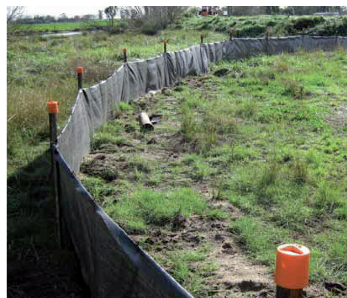
Silt fences are used to limit silt from entering the surrounding waterways
