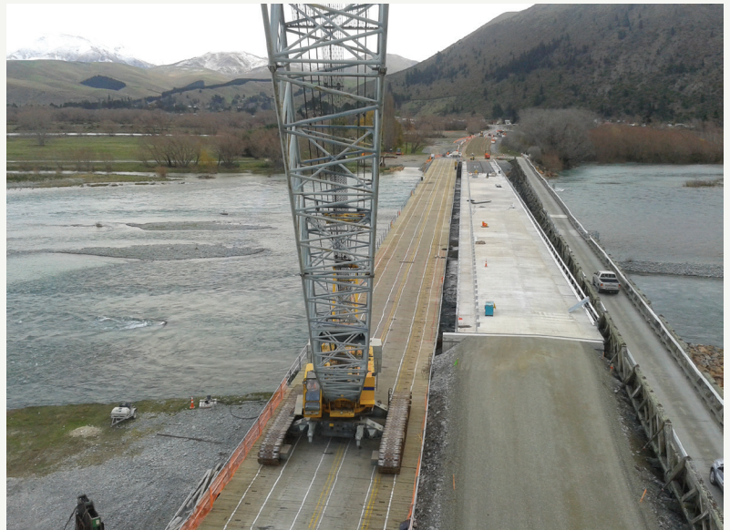
Preparing for the pouring of the final stage of the concrete deck for the new No 1 Bridge
