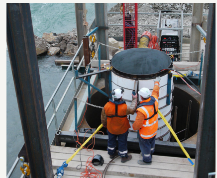
Inspection work on one of the two columns required for Bridge 2 on the Kurow side of the Waitaki River.
