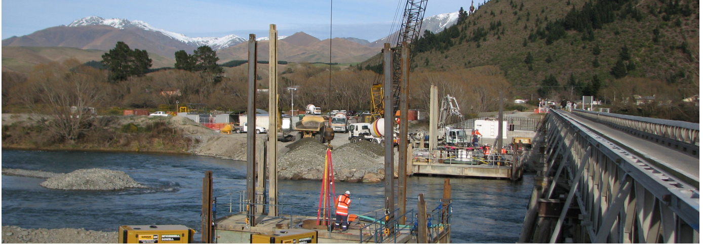
Piling work on Bridge 2 on the Kurow side of the Waitaki River
