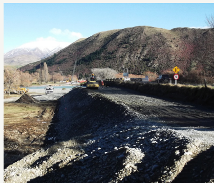
Embankment fill for the approaches to Bridge 1 on the Hakataramea side of the Waitaki River.
