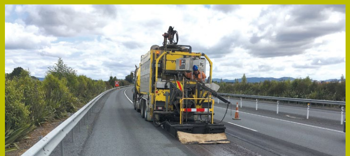
Sealing work at Te Rapa started in February and is nearly finished.
