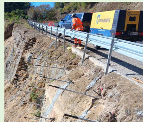
Ground anchors installed and ready for the next stage of the process at Devil's Elbow, SH2
