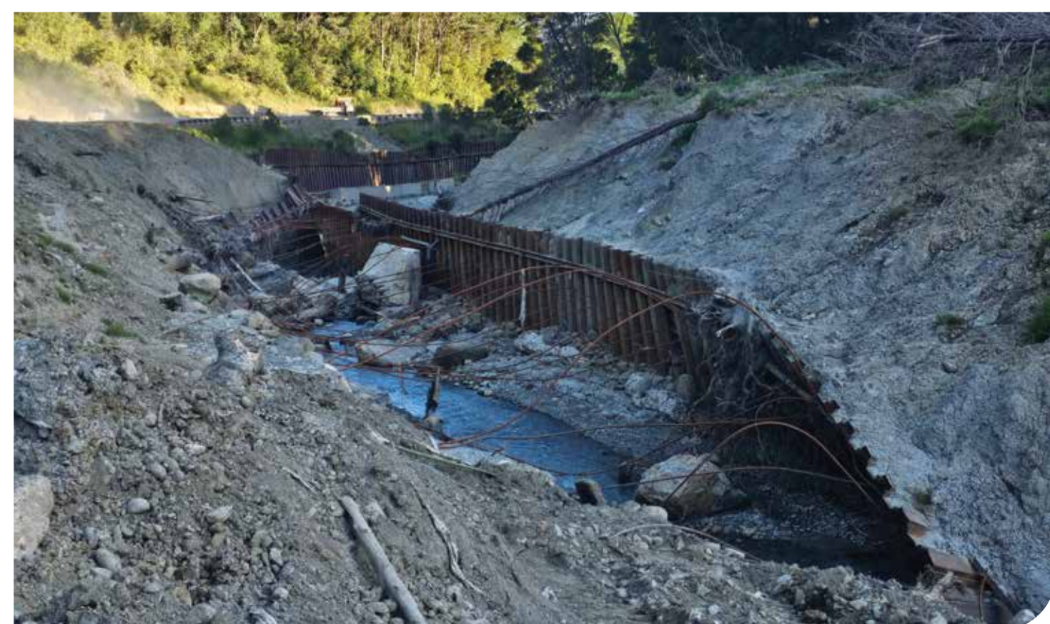
Damage at Mangahauini Gorge
