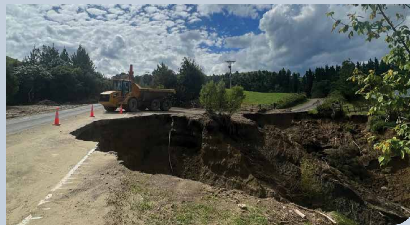
Damage to SH5 following Cyclone Gabrielle
