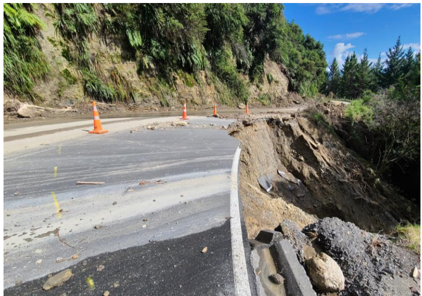
Photo: Cyclone damage at Devil's Corner, March 2023.
