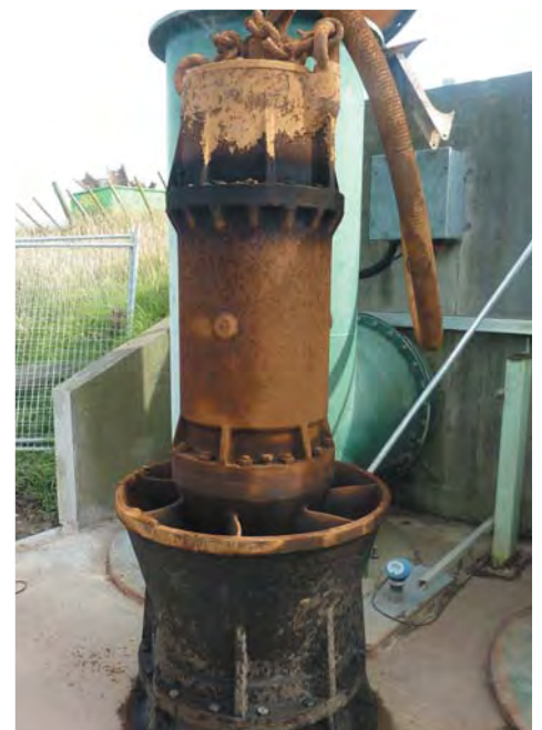
One of the three existing Kaituna pumps out for maintenance. When in operation each can pump 1.5 cubic metres of water per second, emptying an olympic sized swimming pool in just over 27 minutes.
