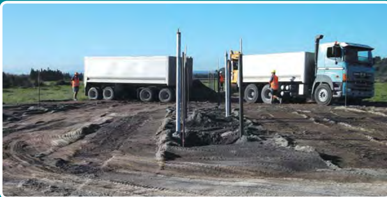
Installing the instrumentation that will capture crucial settlement data. Fill material is then delivered to construct the trial embankment.
