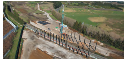
ECMT rail bridge - a total of 32 piles will be driven 30 metres into the ground
