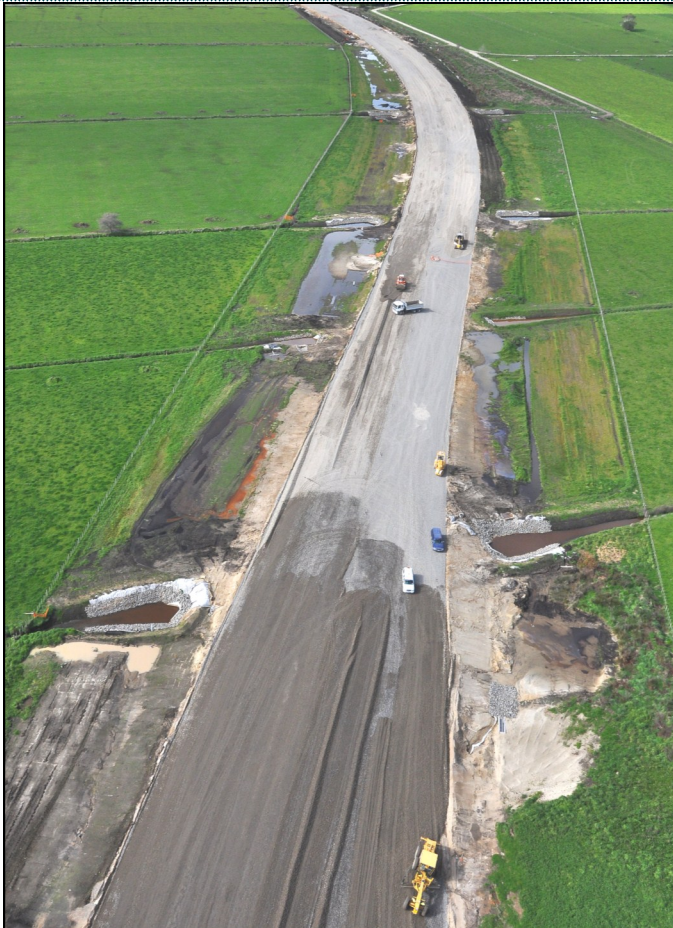
Above: Aerial view of aggregate being placed between Domain Road and Parton Road
