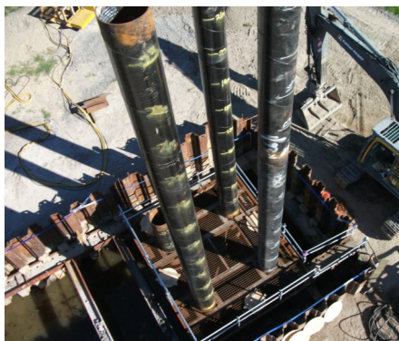
View from above of three casings ready to be driven the first 23 metres
