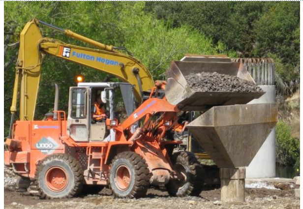
Rock being placed in the ground to create a stone column—photo courtesy East Taupo Arterial project
