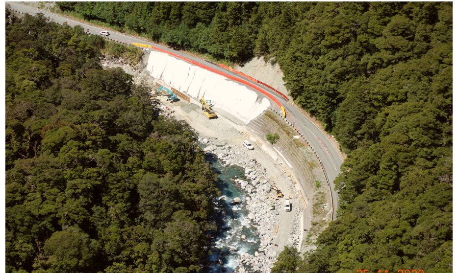
Highway retaining wall repair work between the Hollyford Valley Road turn-off and the Homer Tunnel.
